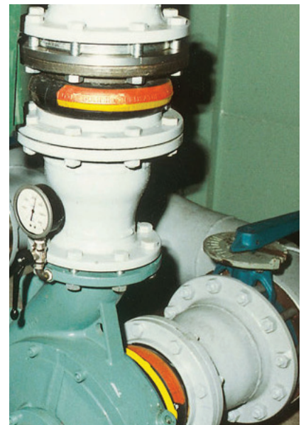
STENFLEX® type AR-1 used at pumps
